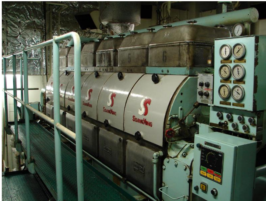
Diesel generator on an oil tanker.
